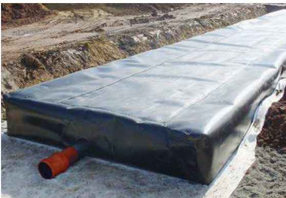
Rainwater tank with foil cover
